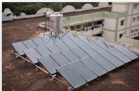
Solar Water Heater – Ladies Hostel 2
