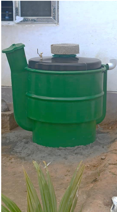
Household Biogas plant
