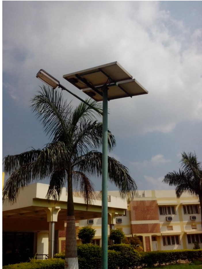
Fig 1. Solar based Street Light
