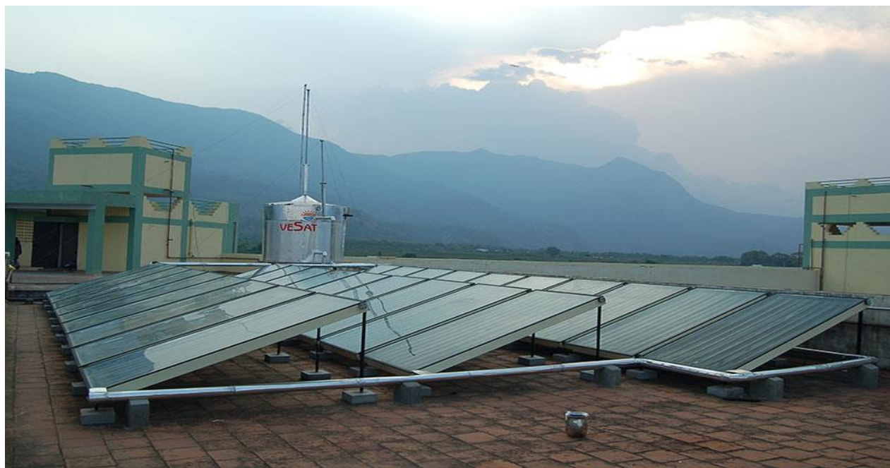
Fig 2. Solar roof top in the Main (Administrative Building)
